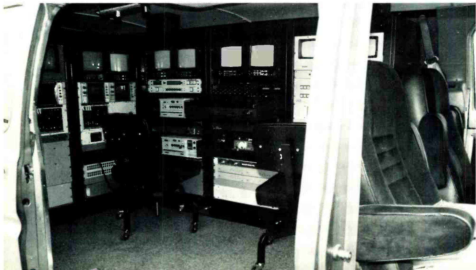
Shook's modification of the Econoline ENG van shows how two-person crew can operate console and video equipment.
